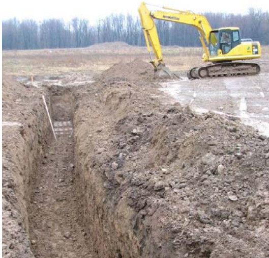
Figure 7. Excavating for the horizontal geothermal loop field. A horizontal installation was selected as a more affordable alternative to a vertical loop field.
