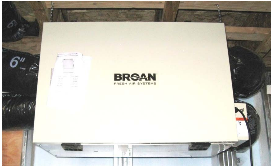
Figure 6. Broan HRV100h for indoor air quality. Note the two 180 degree bends in the supply and return ducts on the right hand side.
